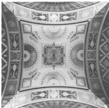
Above and to the left: Interior photographs showing the sumptuous plaster and paint decorations at the Pantages Theatre (photos: Cineplex Odeon Corp.)
